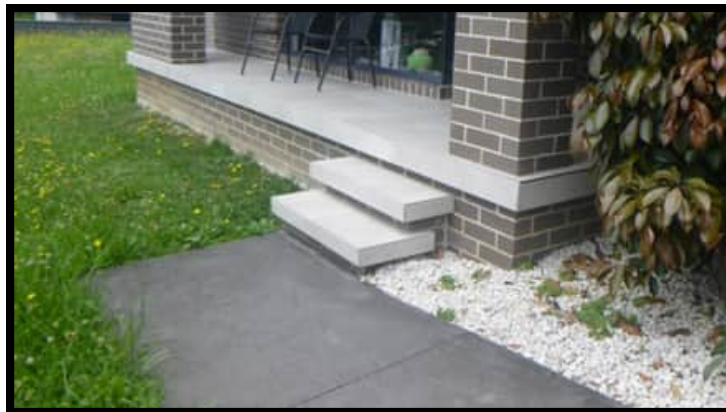
PHOTO B: Same stairs following the installation of the pathway and the tiling of the porch and stairs. The path at the base of the stairs affected the bottom riser height and the tiling changed the heights taking them outside the allowable variations requiring the retiling of the area.
